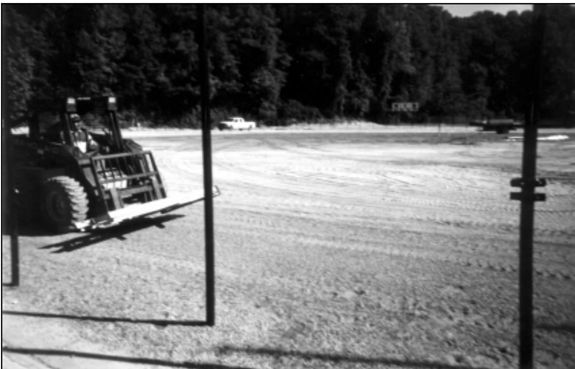
Bulldozers level the playing fields as North Atlanta's athletic fields undergo renovation.
